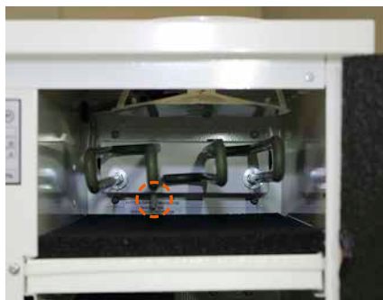
Reset button for the thermal overload cutout on the preheating air heater
