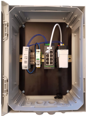
Fig. 6. INSIDE Connect in electrical cabinet with switch.
