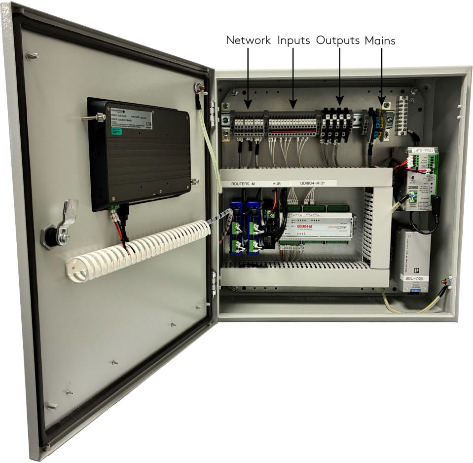
Figure 4. Wiring Inside the Control Panel
