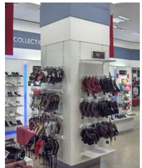
Air diffusers incorporated into retail product display columns save floor space.
